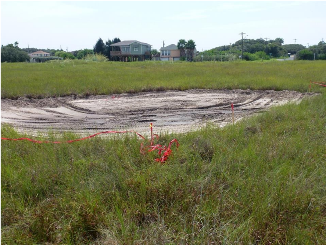
Photo 15. The riparian woodland plot was excavated to the surface of the groundwater table.
